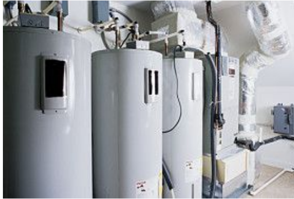
Photo 3 Water Heaters (source, Getty Images)
