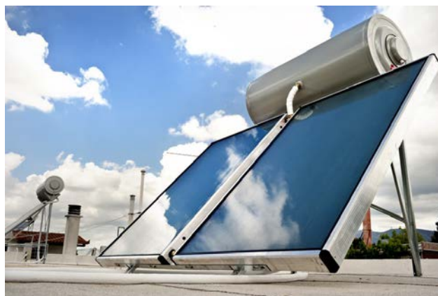
Photo 4 Roof solar heating system (souce, Antonis Liokouras/Getty Images)
